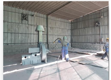
Cement Company Filter System
